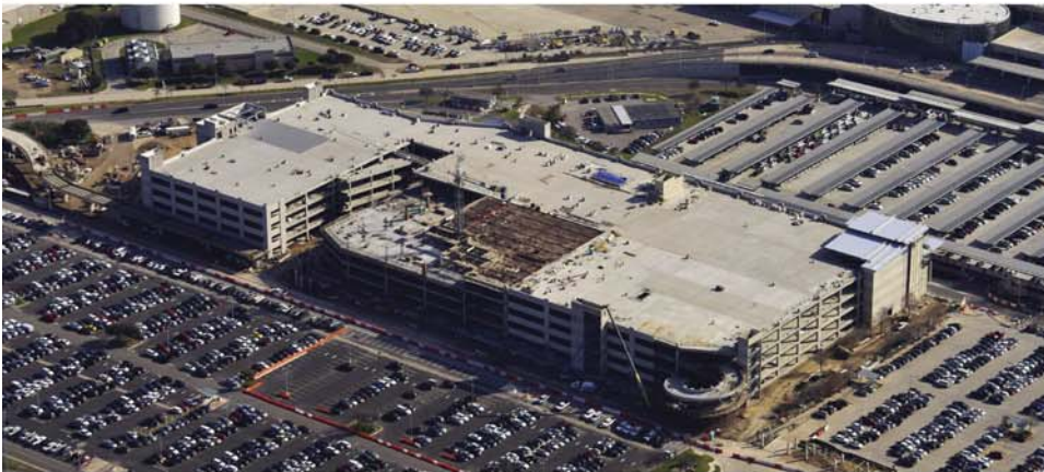
This aerial view shows the construction of the consolidated car rental facility at Austin-Bergstrom International Airport as of Jan. 15, 2015.
